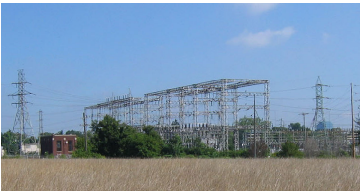
Consumers Energy owns the transmission lines that traverse the site (top), as well as the Wealthy Street electric substation located adjacent to the site (bottom).
